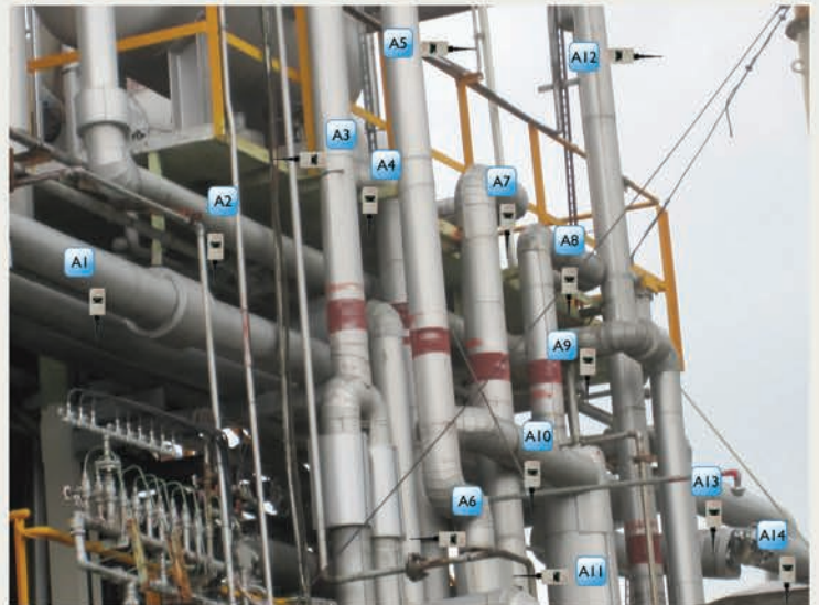
CUI Warning System for Entire pipeline
